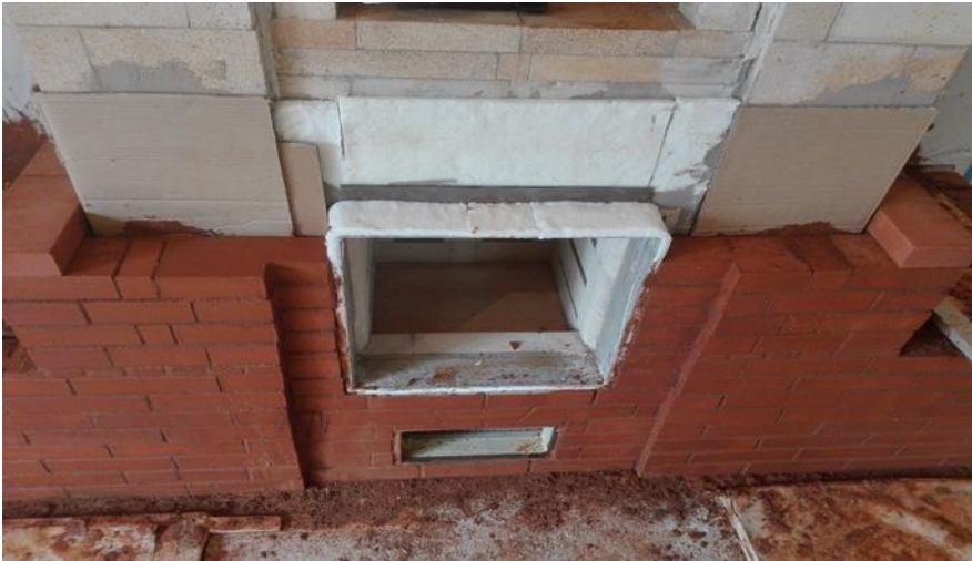
Figure 9: The entire 'Core' of the heater is completed prior to facing the heater. Note: clean outs are visible on the side of the bench as well as below the firebox and above the oven.
