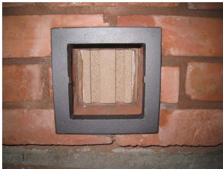
Figure 7: Cast iron clean out frame door not attached)- fire brick plug in core.
